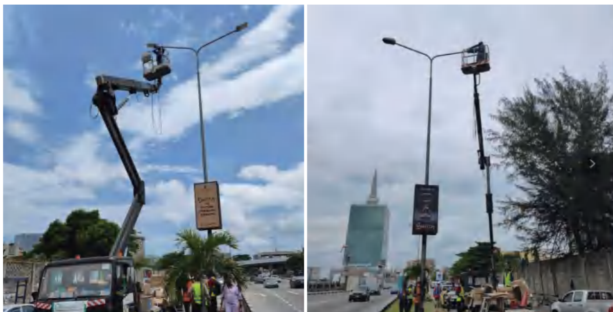
Location: Nigeria Solution: RF-Mesh Quantity: 50,000 sets
